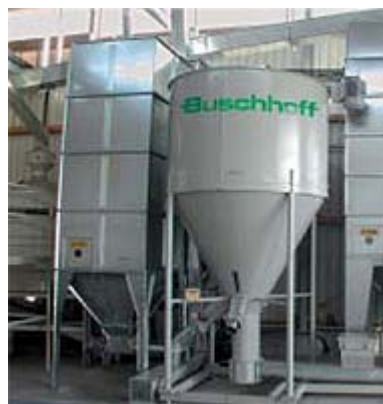
Mill and Mix plant with a GM type feed mixer.
